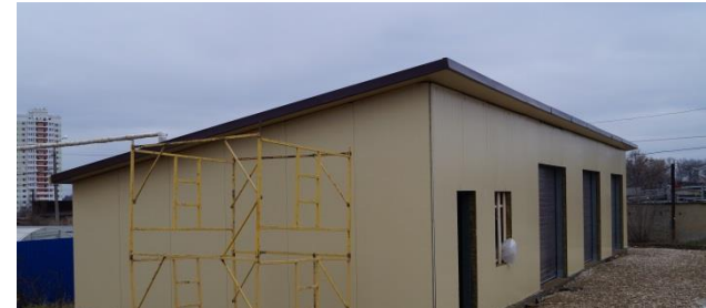
№6. The steel building is ready. It is time to start mounting gates, doors and windows.
